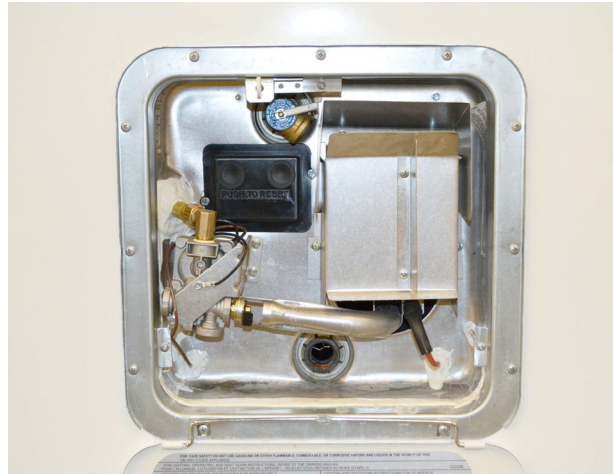
Water Heater Exterior Service Access
