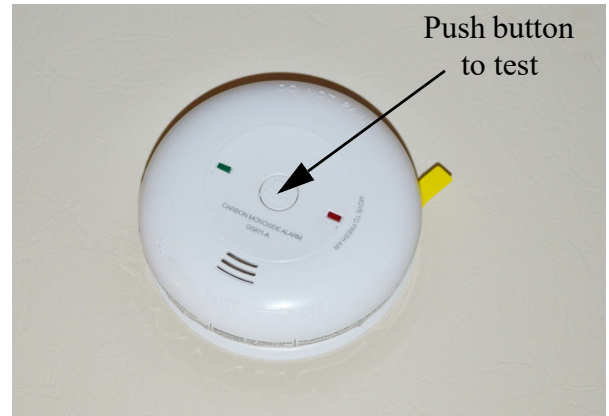
Carbon Monoxide Alarm
