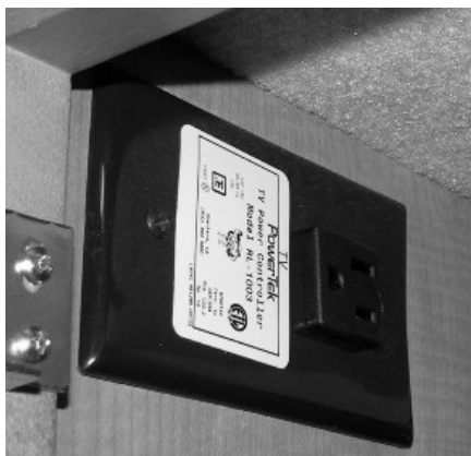
Front TV Ignition Switch Interlock -Typical View
