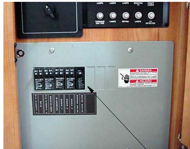
120-Volt House Circuit Breakers
