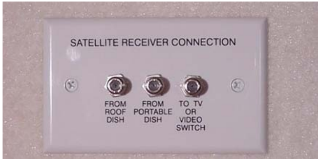
Interior Connection for Satellite Dishes (in cabinet near TV*)
