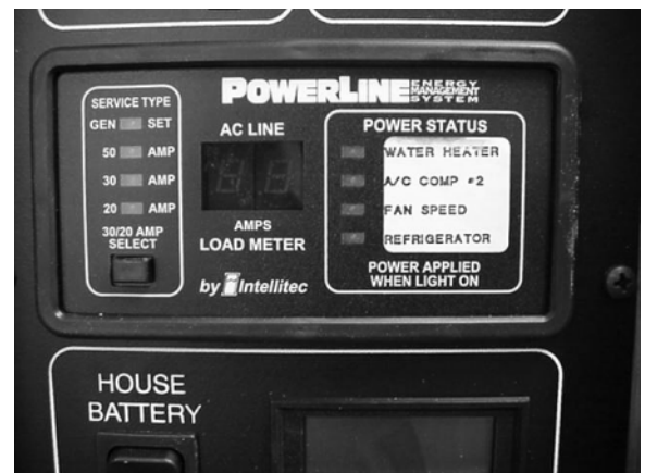
EMS Display on Monitor Panel -Typical View
