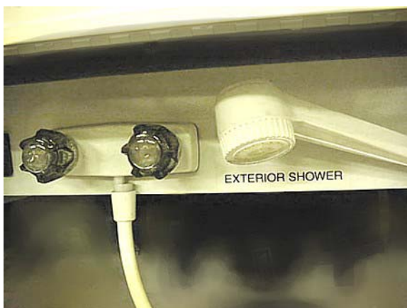
Exterior Shower/Wash Station -Typical View
