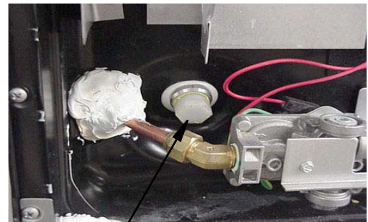
Water Heater Drain Plug Remove with socket
