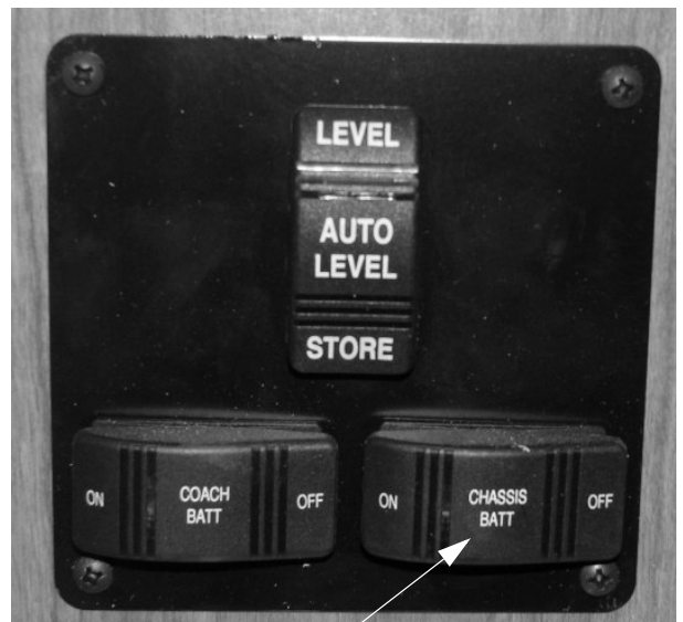
Chassis Battery Disconnect Switch (located inside the entrance door)
