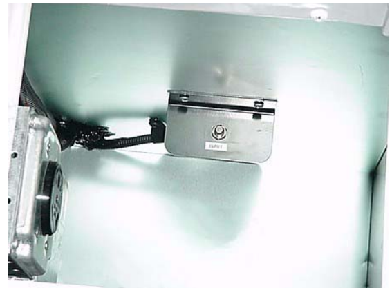
Cable TV Hook-Up in Utility Compartment
