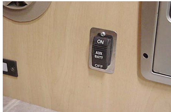
Aux. Batt. Switch - typical (Near entrance door)
