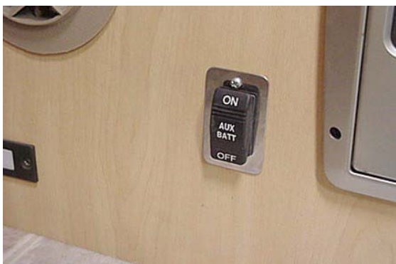
Aux. Batt. Switch - typical (Near entrance door)
