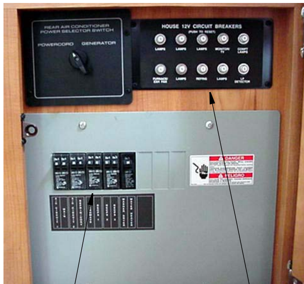
120-Volt House Circuit Breakers
