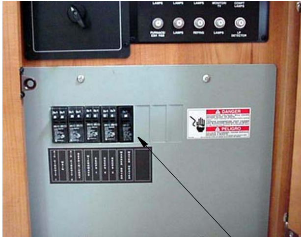
120-Volt House Circuit Breakers
