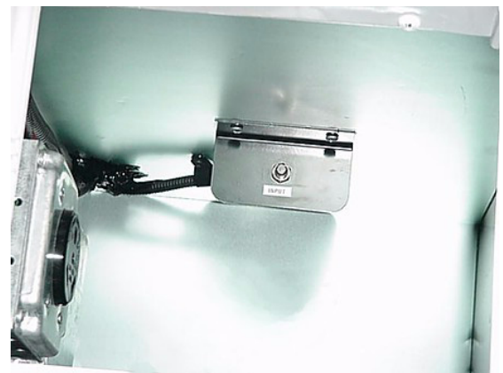
Cable TV Hook-Up in Utility Compartment
