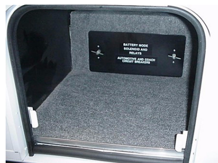
Chassis and House 12V Circuit Breakers behind cover panel in cargo compartment near entrance door
