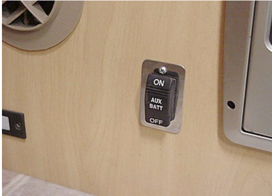
Aux. Batt. Switch (Near entrance door)
