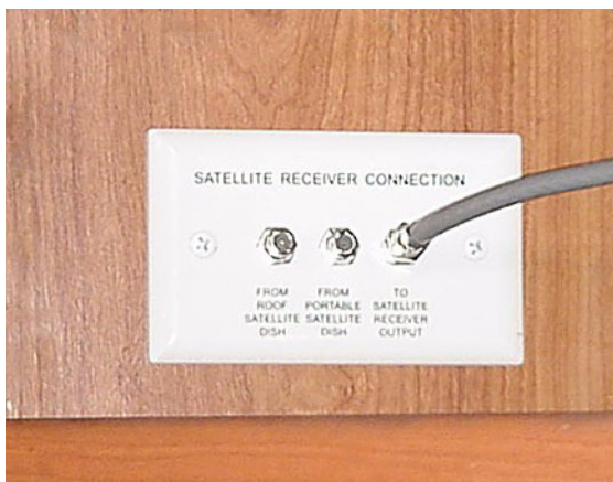
Interior Connection for Satellite Receiver
