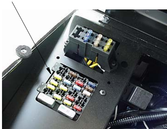
Automotive 12-Volt Fuse Block (Under lift-up dash pod)
