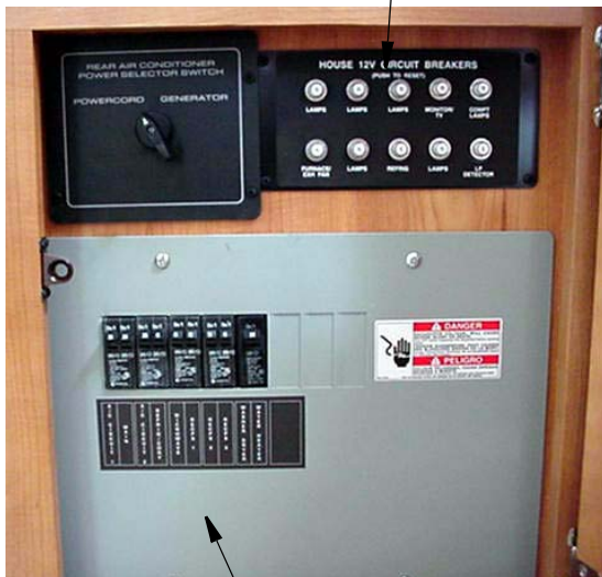
110-Volt Circuit Breakers
