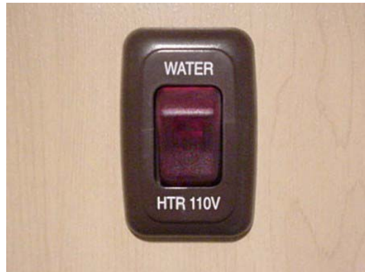
Electric Water Heater Switch (Typical)
