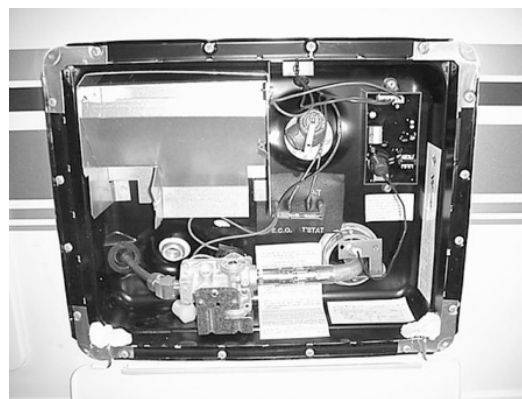
Water Heater Exterior Service Access
