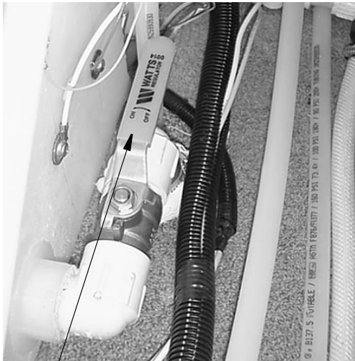
Water Tank Drain Valve (Typical)
