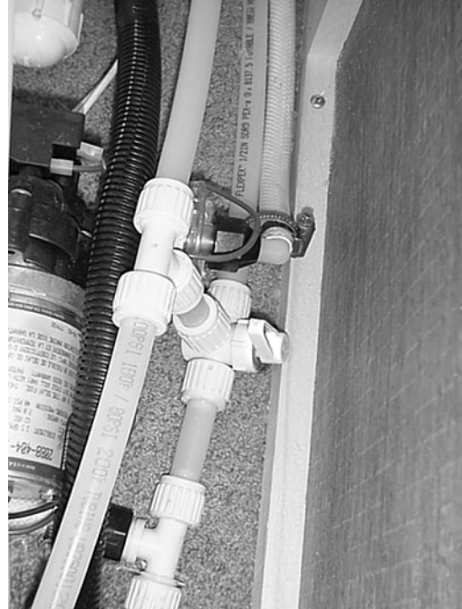
Water Heater By-Pass Valve (Typical)
