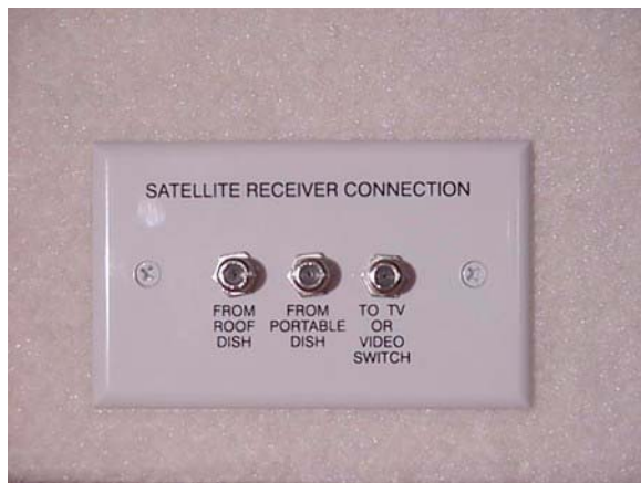
Interior Connection for Satellite Receiver (in video center cabinet)
