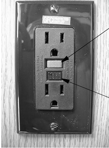
GFCI Outlet (Ground Fault Protector)
