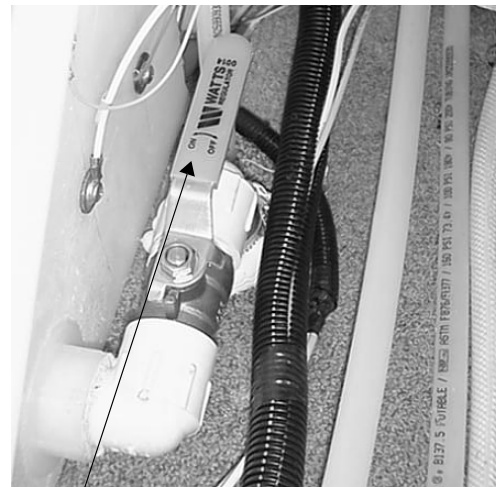
Water Tank Drain Valve
