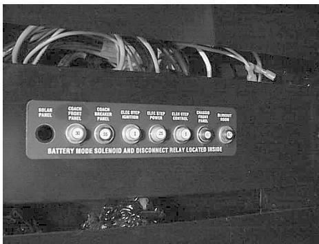
Chassis and House 12V Circuit Breakers behind cover panel in cargo compartment near entrance door
