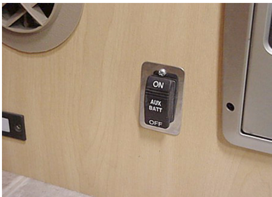
Aux. Batt. Switch (Near entrance door)
