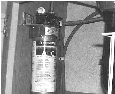
Water Filter Assembly - Below Galley Sink
