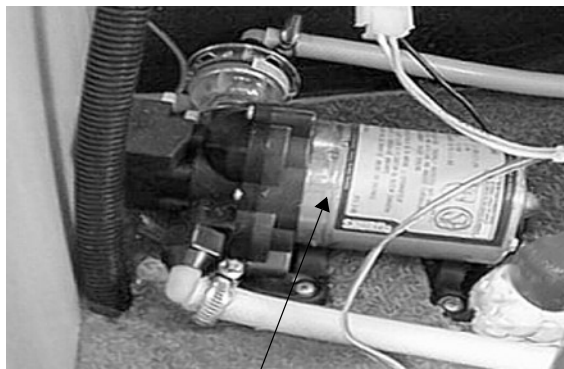
Water Pump (typical)
