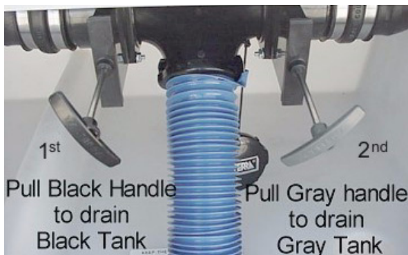
Holding Tank Valves (Typical)
