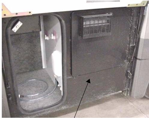
Water Pump Access Panel (typical)
