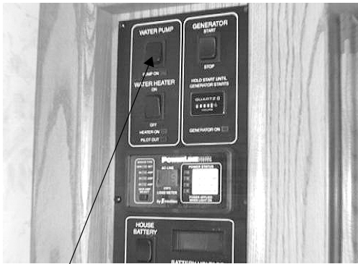
Water Pump Switch
