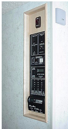
One Place Monitor Panel
