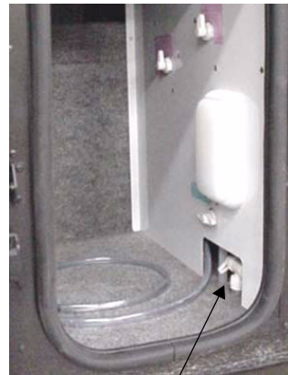
Water Line Drain Valve
