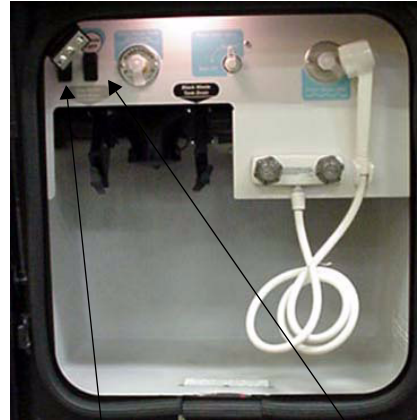
Utility Light Switch
