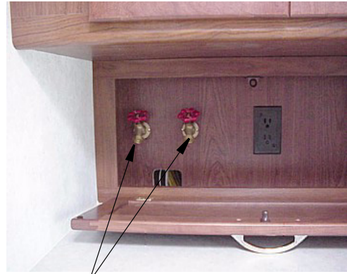
Water Supply Faucets -typical
