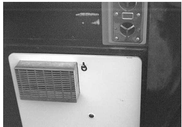
Water Heater Service Access Panel
