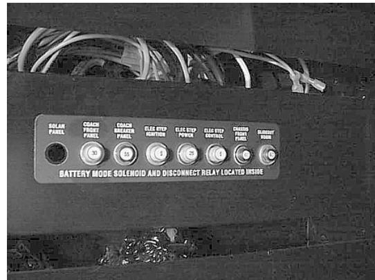
Auto Chassis 12-Volt Breaker Panel
