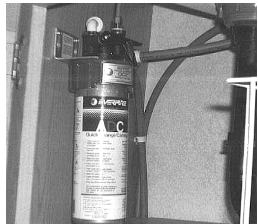
Water Filter Assembly - Below Galley Sink
