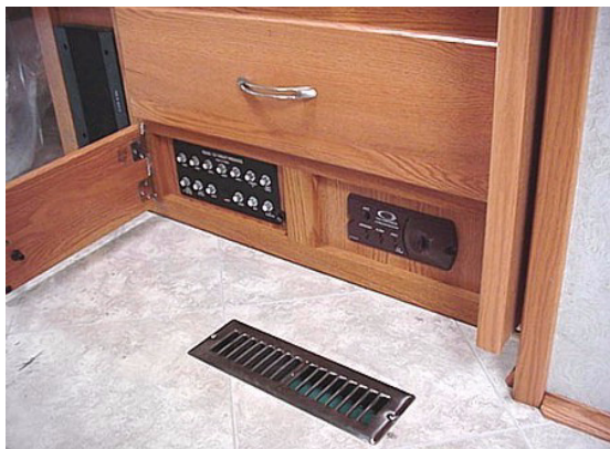
House 12V Breakers (below refrigerator)
