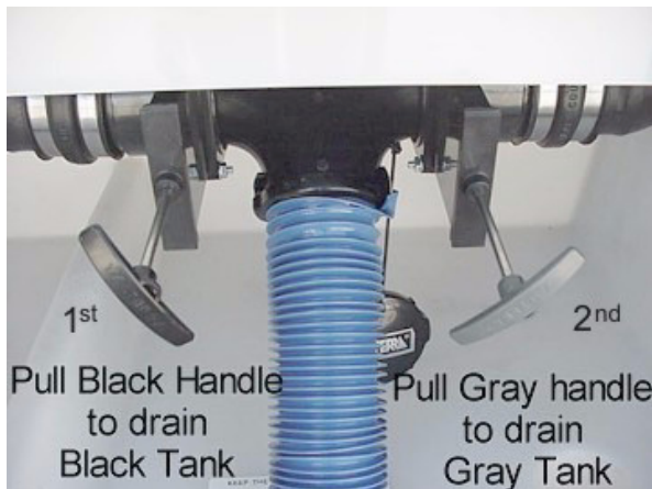
Holding Tank Valves (Typical)
