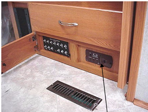
LP Gas Alarm
