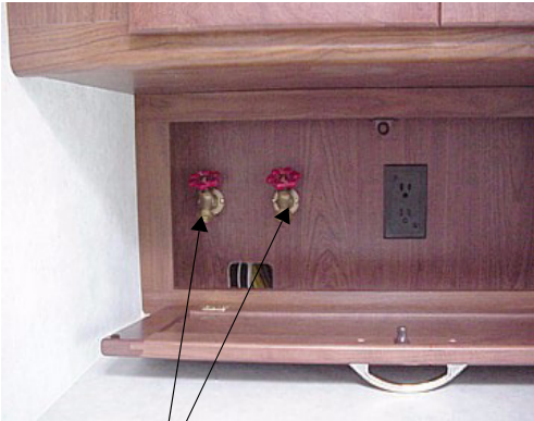
Water Supply Faucets Typical
