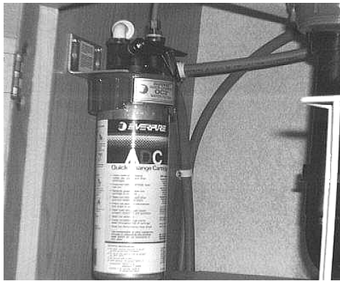
Water Filter Assembly - Below Galley Sink
