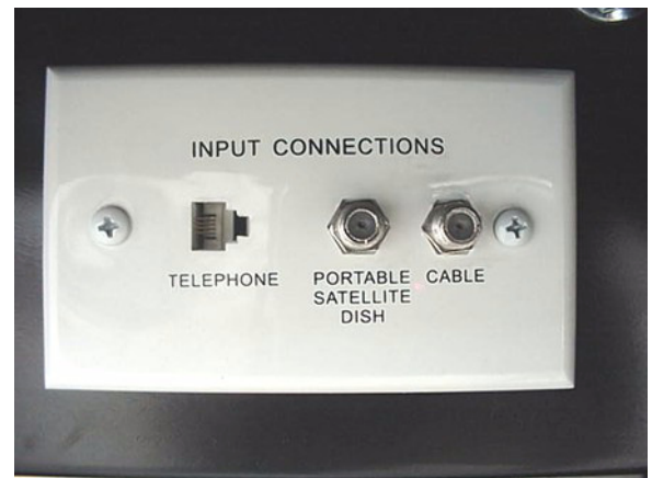
Exterior Connection for Satellite Dishes and Cable TV (In Water Center or Shoreline Compartment)
