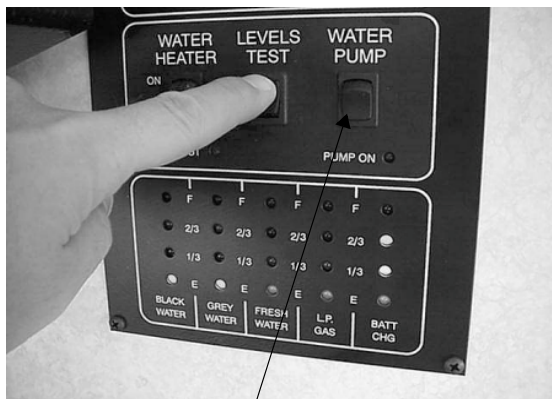
Water Pump Switch
