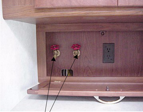
Water Supply Faucets Typical
