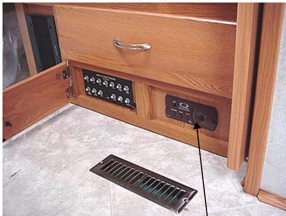
LP Gas Alarm
