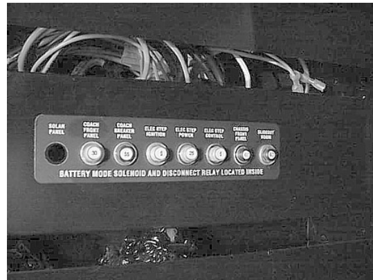
Auto Chassis 12-Volt Breaker Panel
