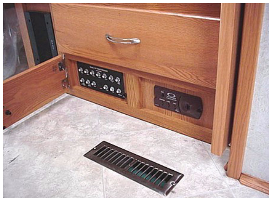
House 12V Breakers (below refrigerator)
