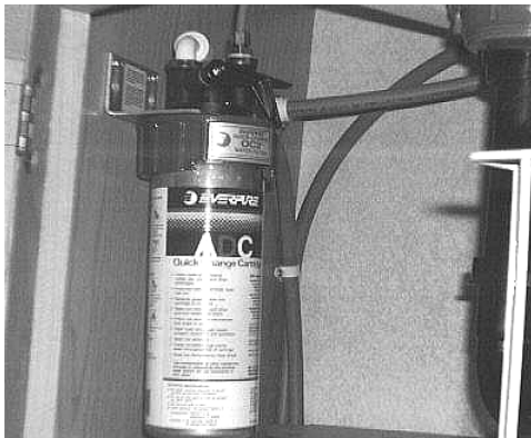
Water Filter Assembly - Below Galley Sink
