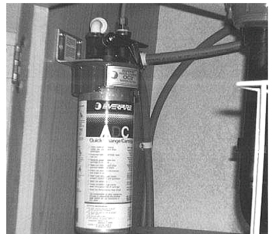
Water Filter Assembly - Below Galley Sink
