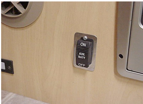
Aux. Batt. Switch (Near entrance door)
