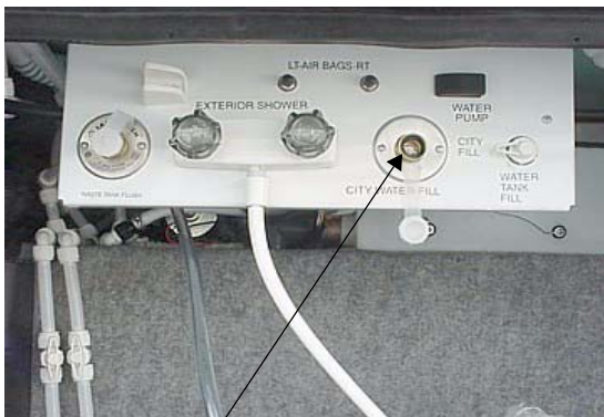
City Water Connection
