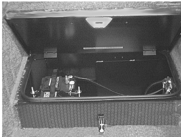
House Battery Storage in Entrance Step
