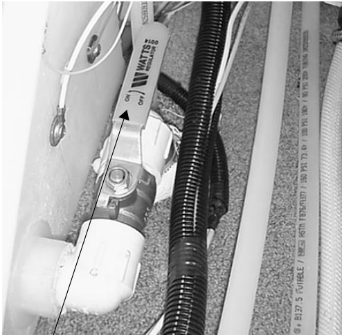
Water Tank Drain Valve
