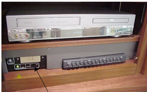
DC-AC Voltage Inverter in Video Center
