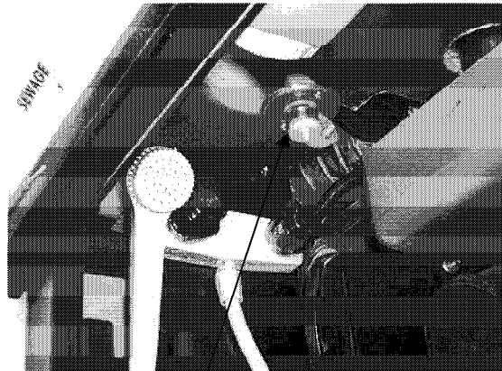
City Water Connection
