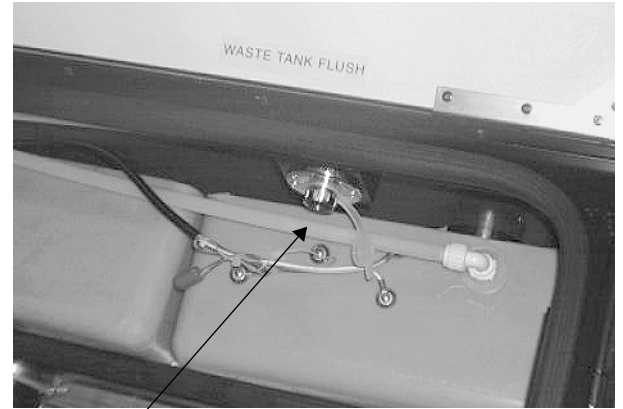
Flushing System Inlet
