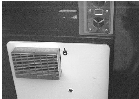
Water Heater Service Access Panel
