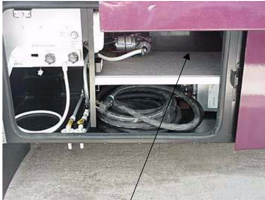
Inverter Charger Unit Location
