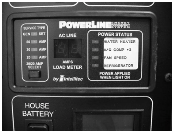
EMS Display on OnePlace Monitor Panel
