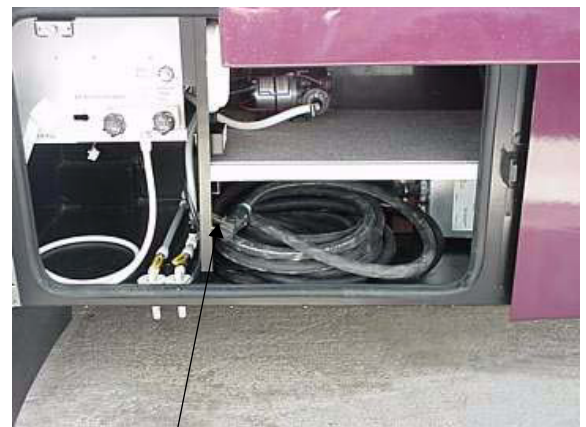
Water Heater By-Pass Valve
