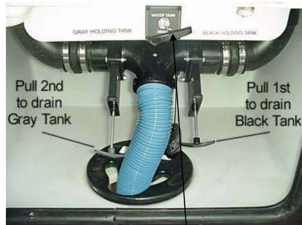
Water Tank Drain Valve (pull to open)
