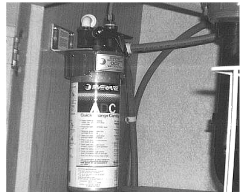
Water Filter Assembly - Below Galley Sink
