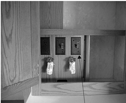
Engine Block Heater Switch (Typical)
