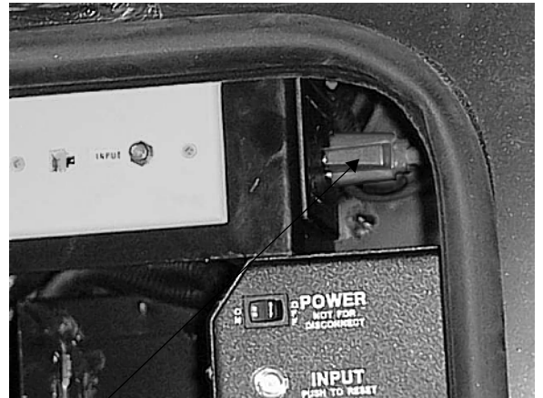
Engine Heater Cord above Inverter/Charger in Shoreline Compartment
