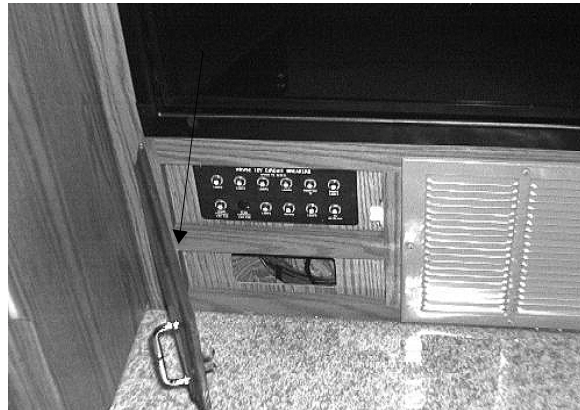
House 12-Volt Circuit Breaker Panel
