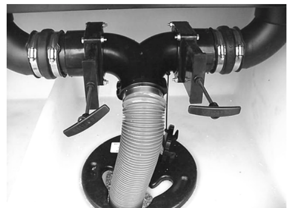
Drainage Hose routed through passage in compartment
