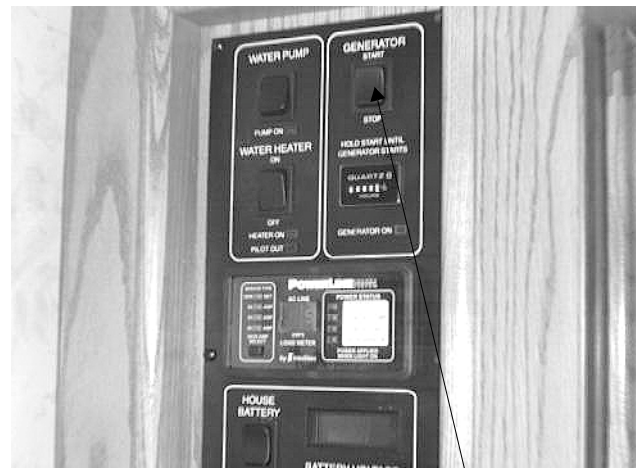
Generator Switch and Hourmeter
