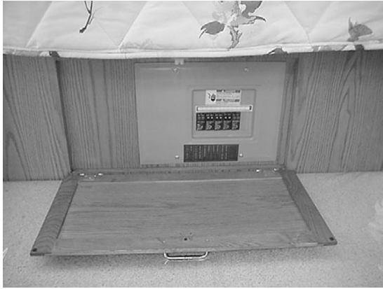
110-Volt House Circuit Breakers (at foot of bed)
