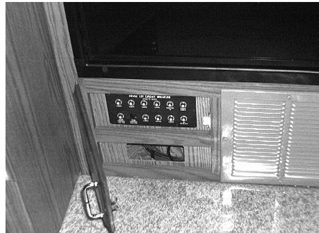
House 12V Breakers (below refrigerator)
