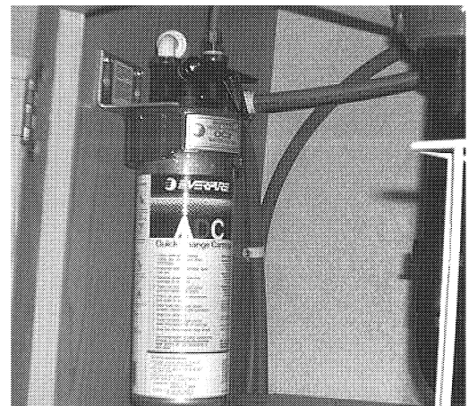
Water Filter Assembly - Below Galley Sink
