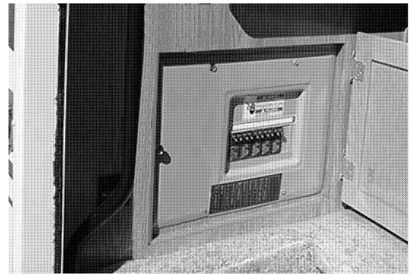
110-Volt Circuit Breaker Panel (Basement Models)
