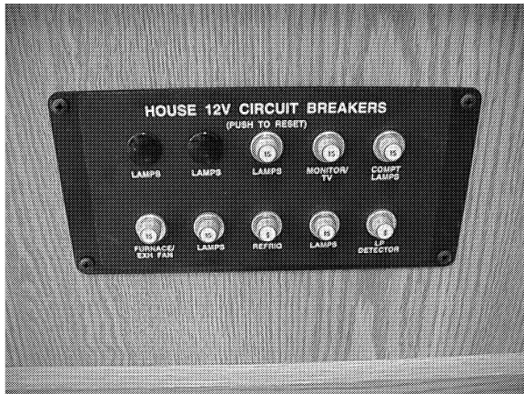
House 12V Circuit Breakers Basement Models
