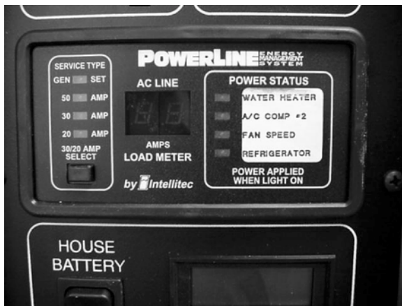
EMS Display on OnePlace Monitor Panel
