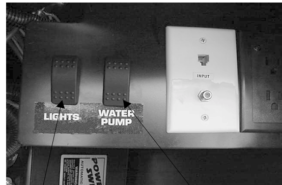
Tank Monitor Panel
