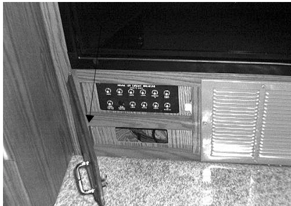
House 12-Volt Circuit Breaker Panel
