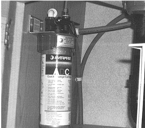
Water Filter Assembly - Below Galley Sink
