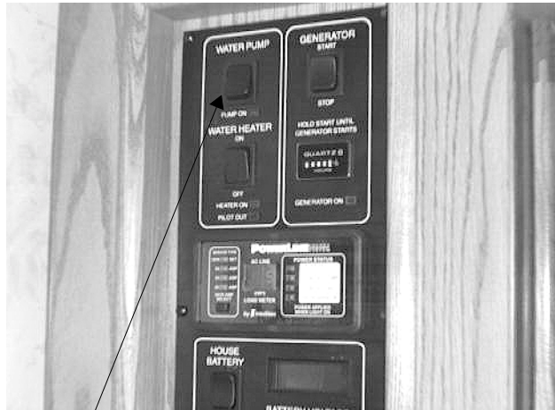
Water Pump Switch
