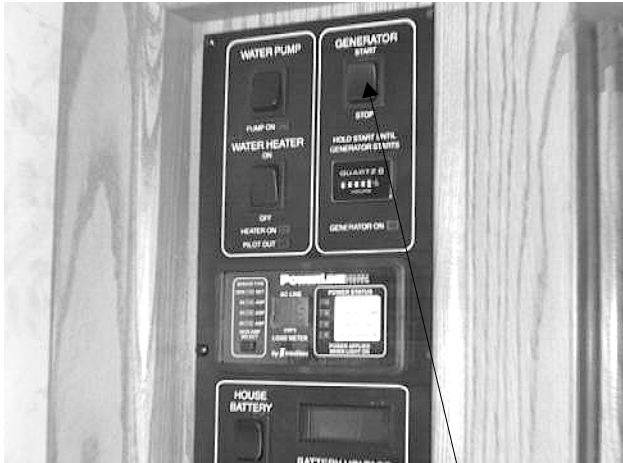
Generator Switch and Hourmeter
