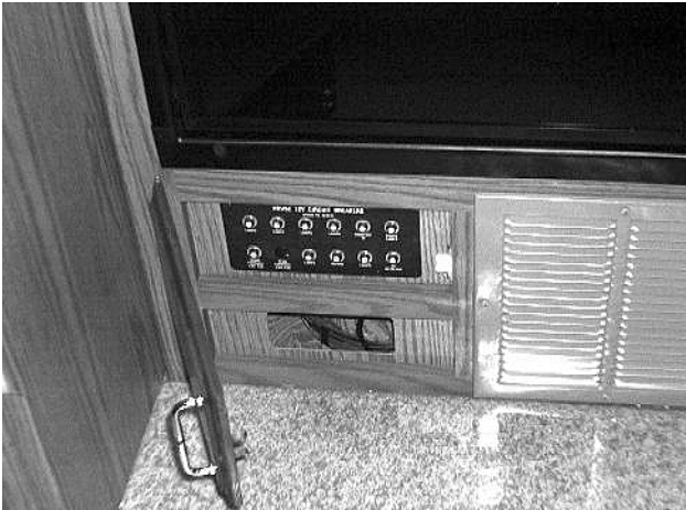
House 12V Breakers (below refrigerator)
