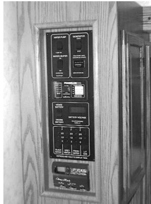
One Place Monitor Panel
