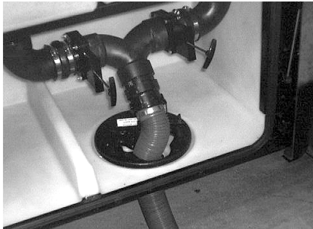
Drainage Hose routed through passage in compartment
