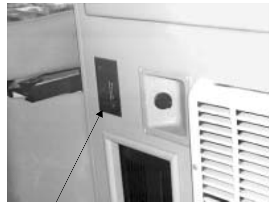
Water Heater Power Switch
