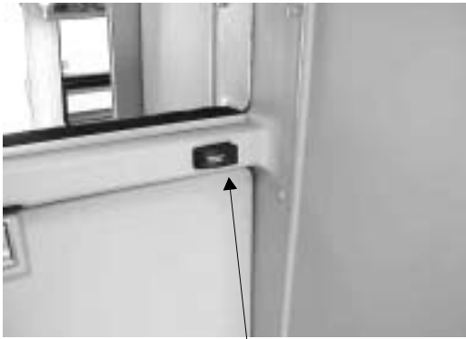
Shower Drain Pump Switch
