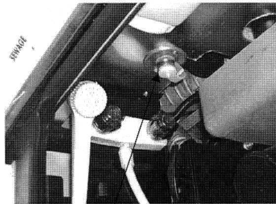
City Water Connection
