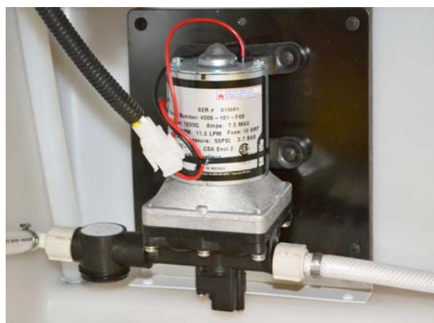
Water Pump -Typical View
