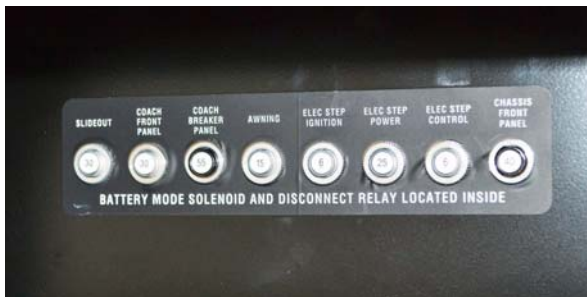
Automotive Chassis and House 12-Volt Circuit Breakers (Located inside passenger compartment) -Typical View
