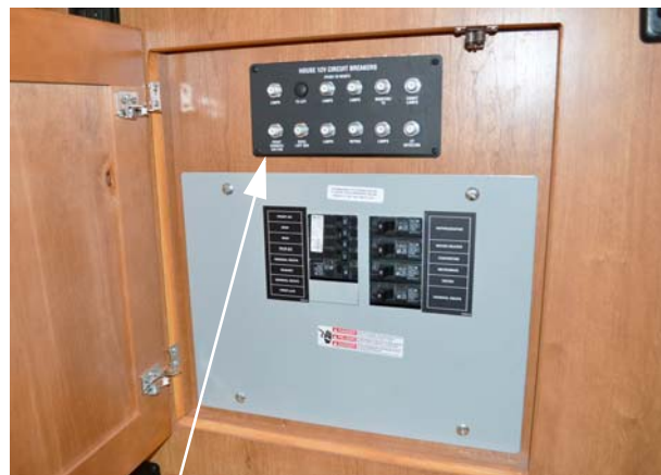
House 12-Volt Circuit Breakers
