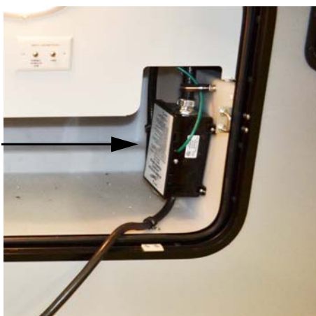
Automatic Power Transfer Box (Located inside water service center compartment) -Typical installation shown
