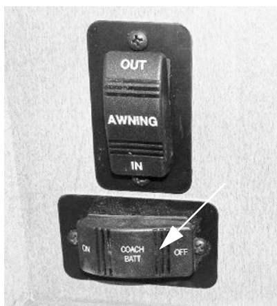
House/Coach Battery Disconnect Switch (Located near entrance door) -Typical View
