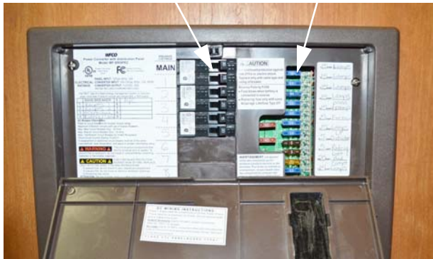
Power Center (Converter) -Typical View
