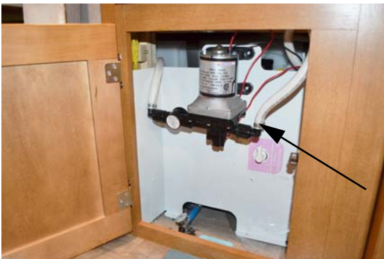
Water Pump (Located behind access door in bottom of pantry) *Models 22M
