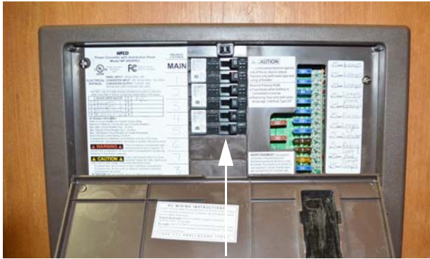
120-Volt Circuit Breakers -Typical View
