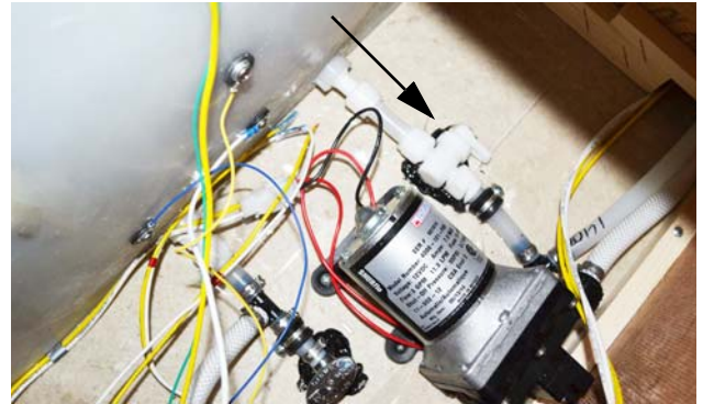
Waterline Drain Valve -Typical View
