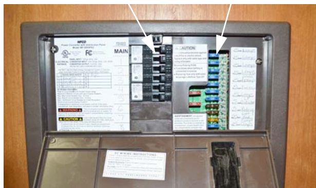
Power Center (Converter) -Typical View
