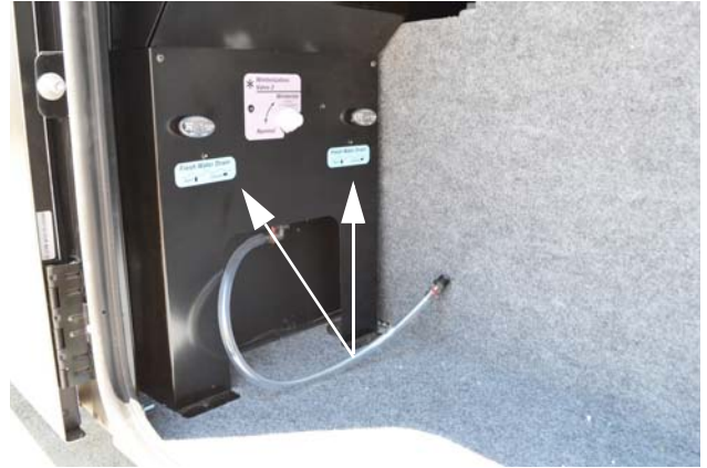
Waterline Drain Valves (Located in the third passenger side compartment) -Typical View
