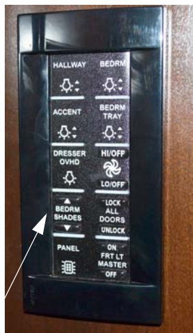
12-Volt Night Shade Switches - Bedroom *Switch located by wardrobe shown. A second switch is located above the bed for your convenience. -Typical View
