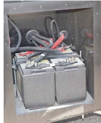
Chassis Batteries (Located behind a rear passenger side exterior door) -Typical View
