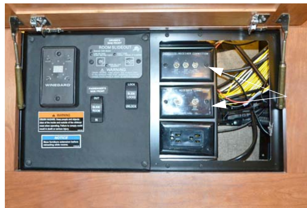
Interior Connections for Satellite Dish (Located in the overhead compartment above entrance door)
