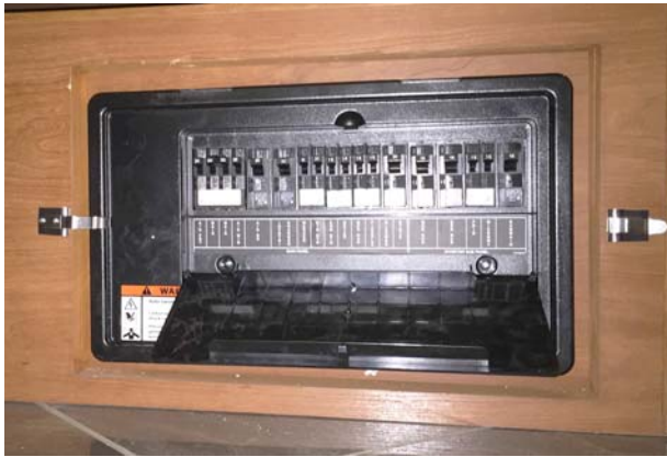
House Circuit Breakers -Typical Installation
