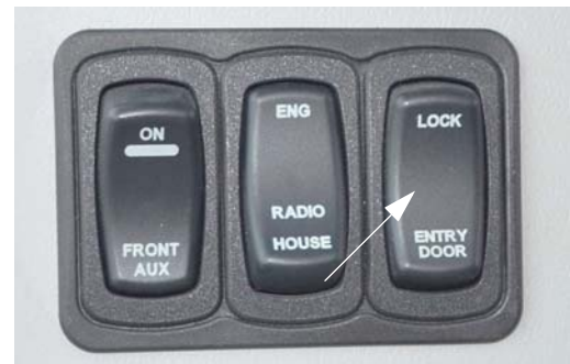
Power Door Locks - Entry Door (Located on dash) -Typical View
