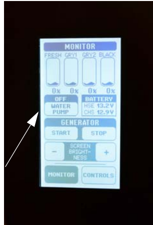
Water Pump Switch (Located on exterior water service center) -If Equipped
