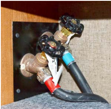
Water Supply Faucets -Typical View
