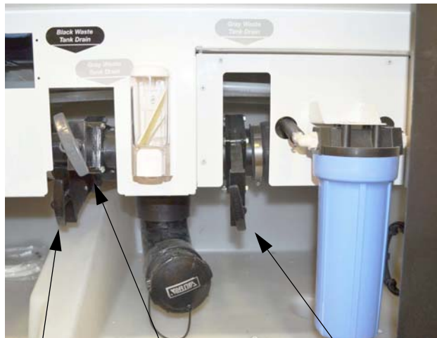
Black Waste Tank Drain Valve Gray Waste Tank Drain Valve #1 Gray Waste Tank Drain Valve #2
