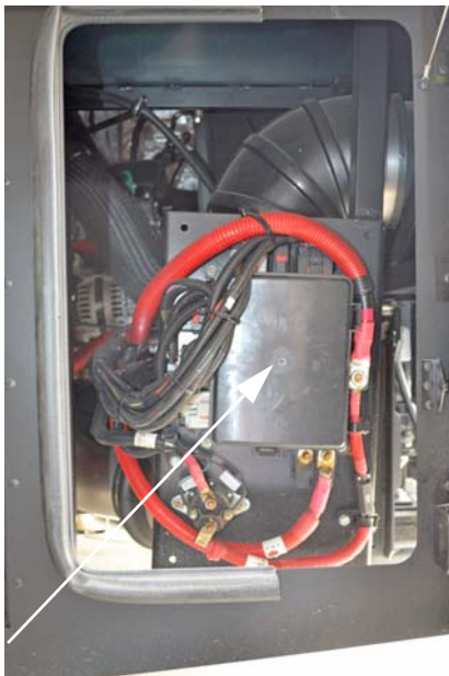
Towing Package Fuses (Located in driver side rear compartment) -Typical View
