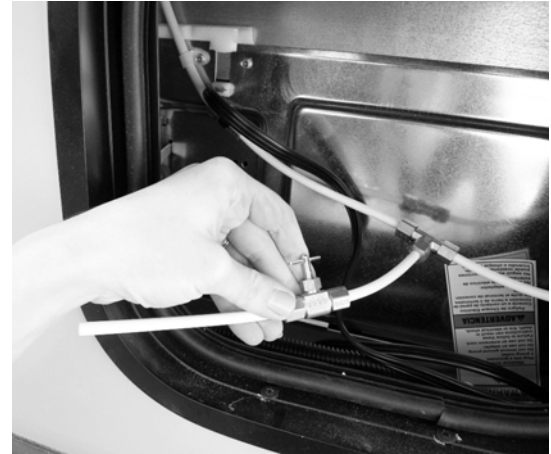
Ice Maker Winterization Drain Valve (Located in exterior Residential Refrigerator service compartment)
