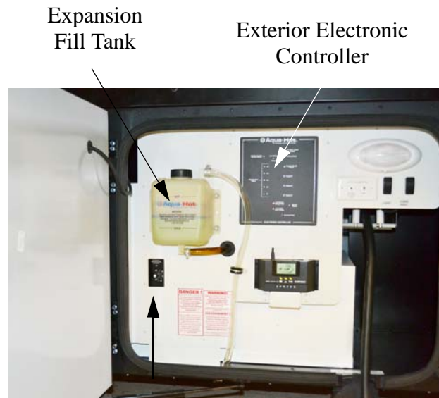
Basement Temperature Control
