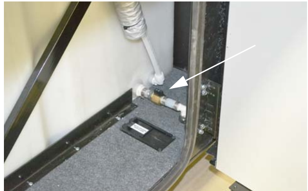
Water Tank Drain Valve (Located in the third passenger side compartment) -Typical View
