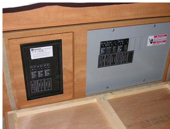
House Circuit Breakers -Typical Installation
