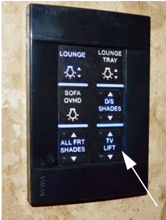
Buffet TV Power Lift/Lower Control Switch (Located near sofa) -Typical View
