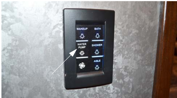
Water Pump Switch (Located in all bath areas)
