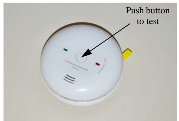
Carbon Monoxide Alarm
