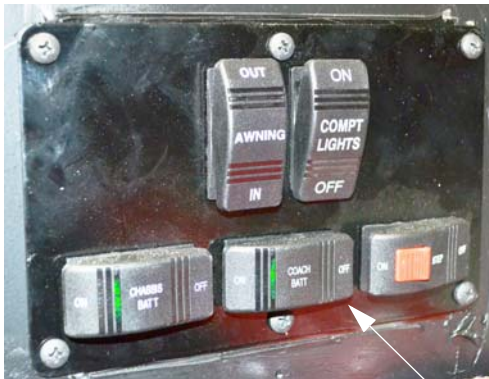
House/Coach Battery Disconnect Switch (Located near entrance door) -Typical View
