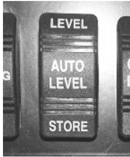
Auto Level Remote Switch (Located near entrance door) -Typical View
