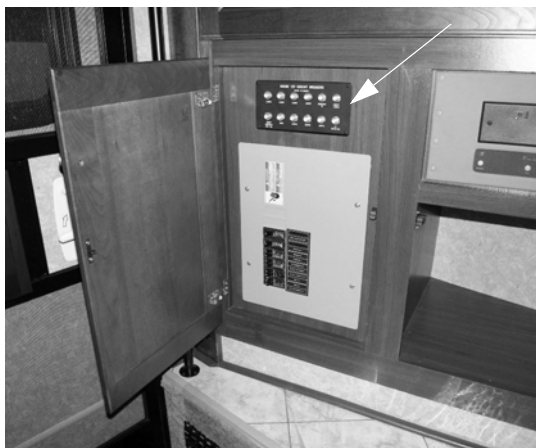
House 12V Circuit Breaker Panel -Typical View
