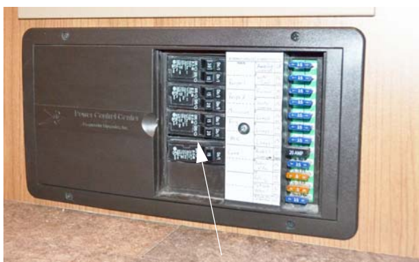
120-Volt House Circuit Breakers -Typical View
