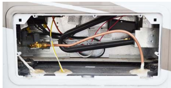
Refrigerator Access Compartment -Typical View
