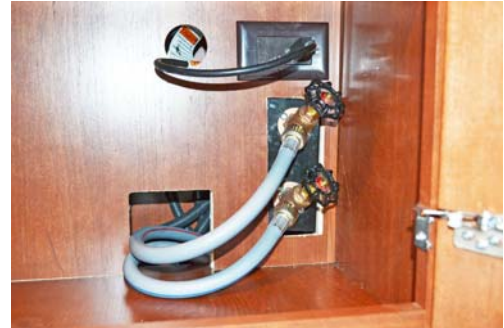
Water Supply Faucets (Located inside cabinet above washer) -Typical View
