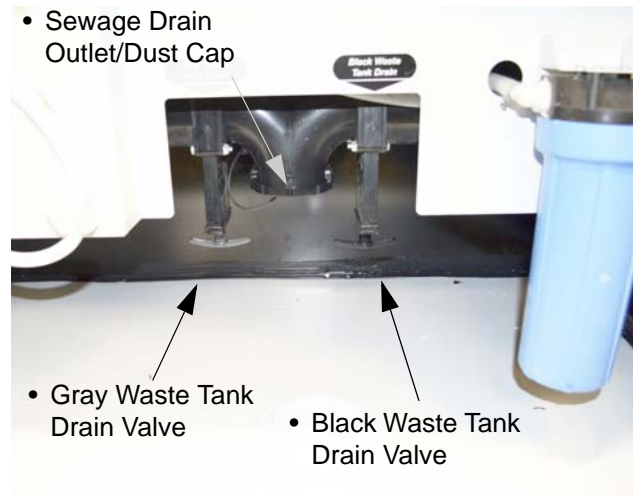
Holding Tank Drain Valves (Located in holding tank compartment) -Typical View
