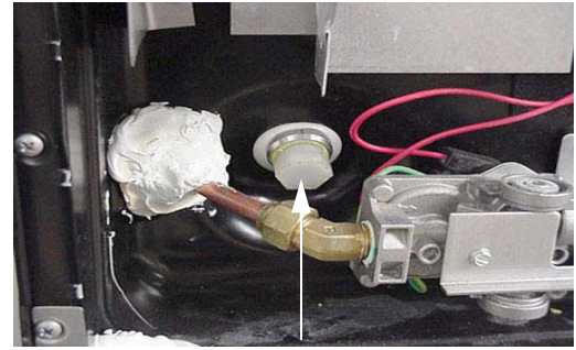
Water Heater Drain Plug (Remove with socket)
