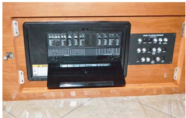
House Circuit Breakers -Typical Installation
