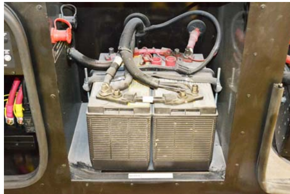
Chassis Batteries -Typical View
