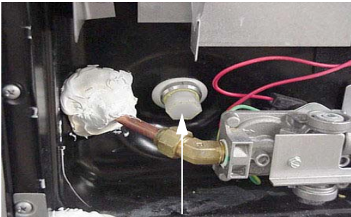
Water Heater Drain Plug (Remove with socket)
