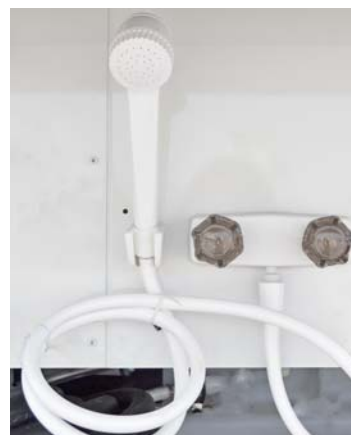
Exterior Shower/Wash Station -Typical View
