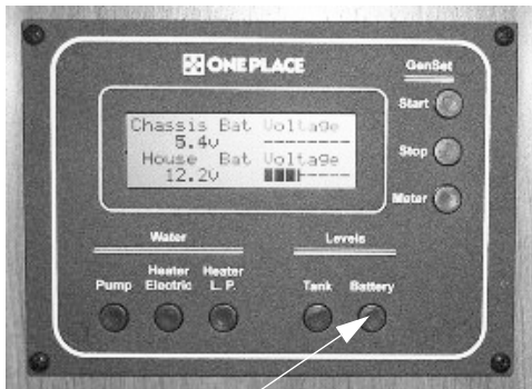
Battery Levels Switch
