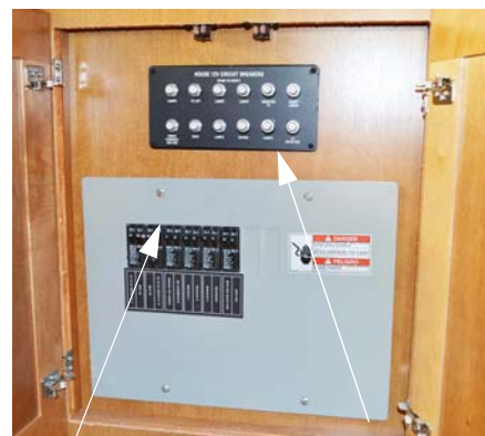
120-Volt House Circuit Breakers
