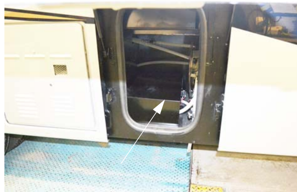
Water Pump (Located inside a passenger side compartment in front of water heater) * Models 32D shown
