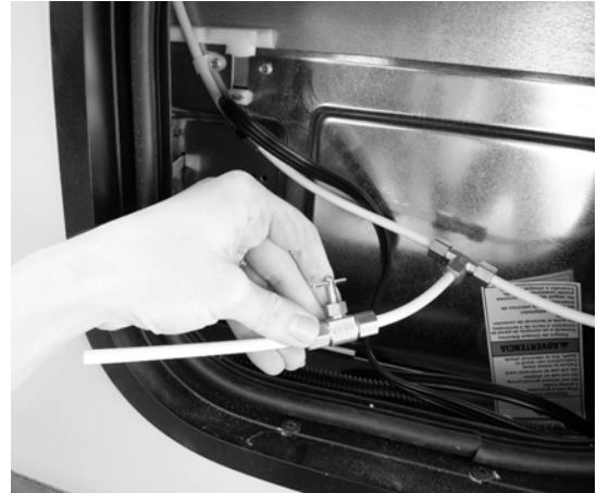
Ice Maker Winterization Drain Valve (Located in exterior Residential Refrigerator service compartment)
