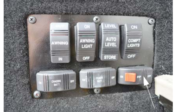
Entry Step Switch (Located near the entrance door) -Typical View
