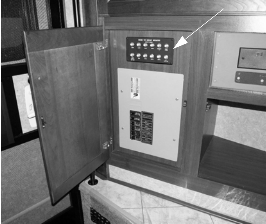
House 12-Volt Circuit Breaker Panel -Typical View
