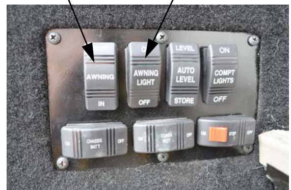
Awning Control Switch and Awning Light Switch (Located near entrance door) -Typical View
