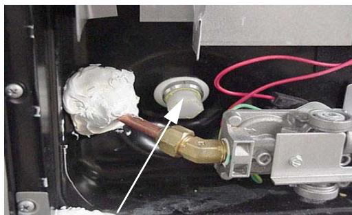
Water Heater Drain Plug (Remove with socket)
