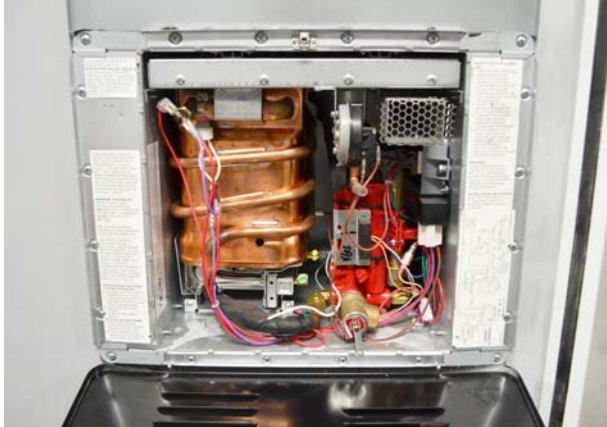
Water Heater Exterior Service Access -Typical View
