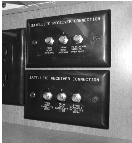
Interior Satellite Dish Connections (Located in the entertainment center cabinet) -Typical View
