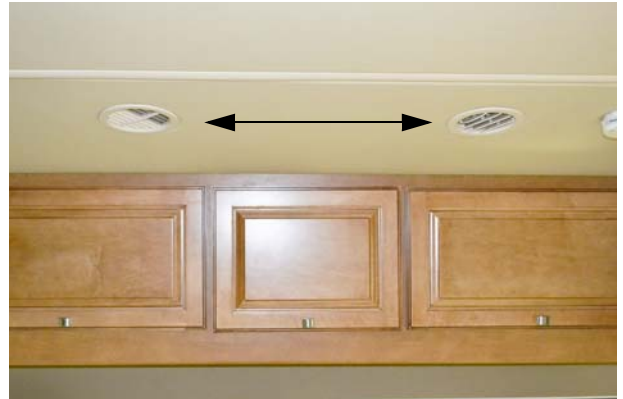
Supply/Return Air Vents (Located throughout the ceiling of the coach) -Typical View
