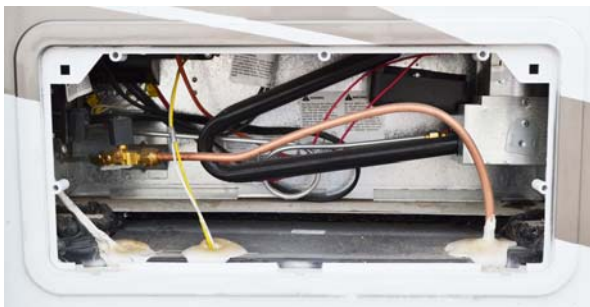
Refrigerator Access Compartment -Typical View
