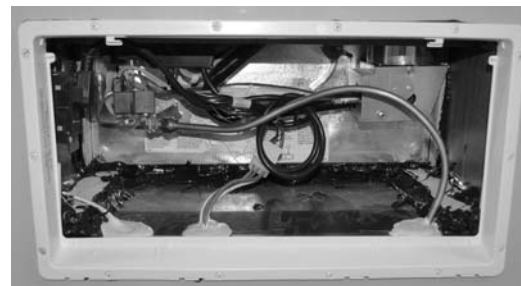
Refrigerator Access Compartment *Shown with cover removed -Typical View
