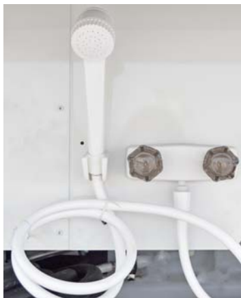
Exterior Shower/Wash Station -Typical View
