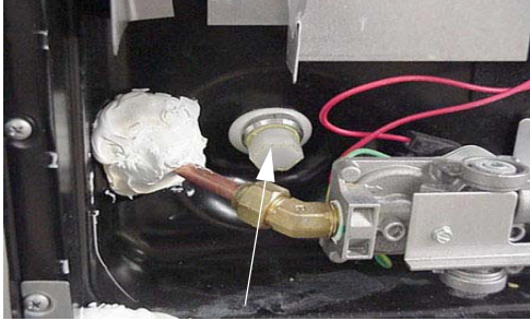
Water Heater Drain Plug (Remove with socket)
