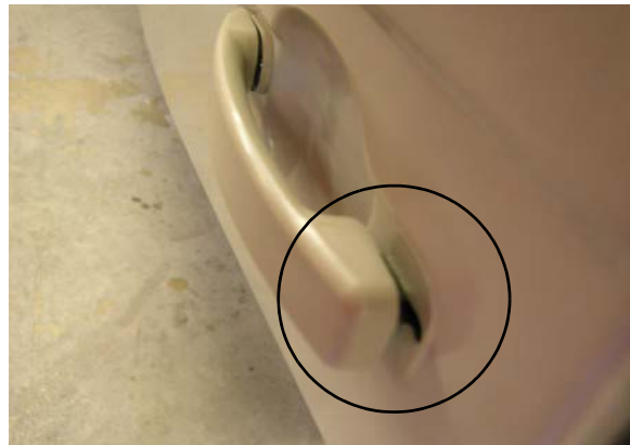
Door Unlatched (note gap)
