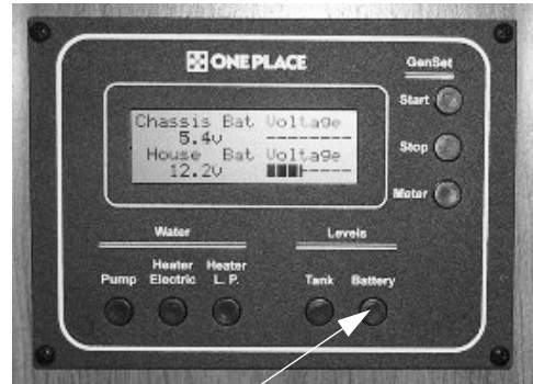
Battery Levels Switch
