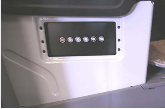
Automotive Chassis 12-Volt Circuit Breakers (Located on outboard side of passenger seat) * Shown with cover removed -Typical View
