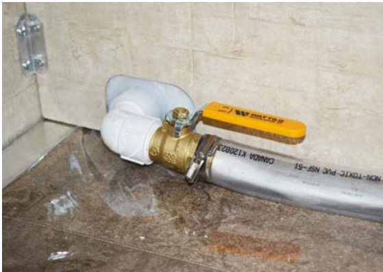
Water Tank Drain Valve ON -Typical installation shown
