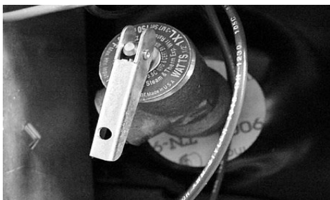
Pressure-Temperature Relief Valve (Lift handle only when water heater is cold)
