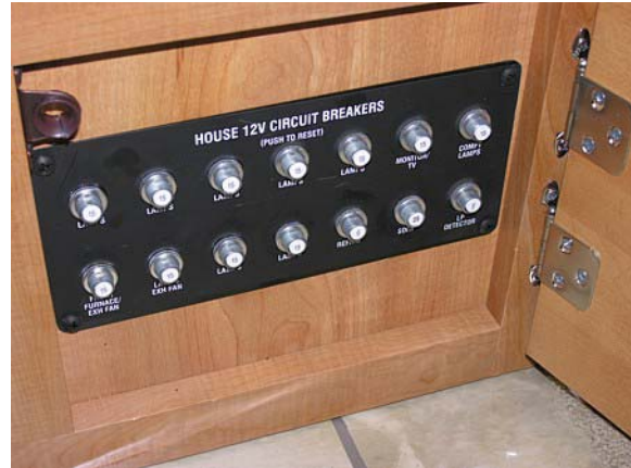
House Circuit Breakers -Typical View
