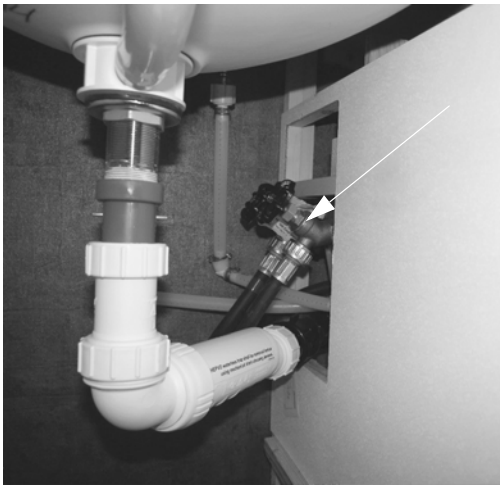
Water Supply Faucets (Located below lavatory cabinet) -Typical View
