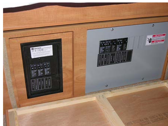
House Circuit Breakers -Typical Installation
