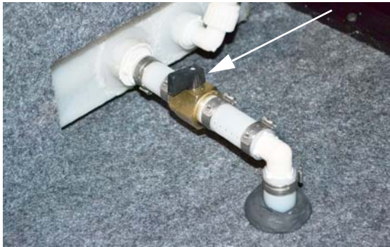
Water Tank Drain Valve (Located in the third passenger side compartment) -Typical View
