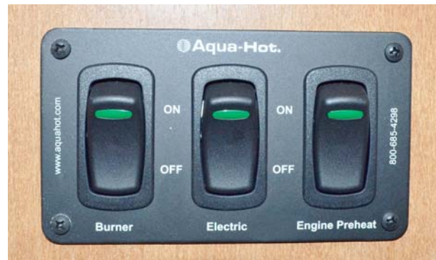
Hydronic Heating System Interior Control Switches (Located near monitor panel) -Typical View
