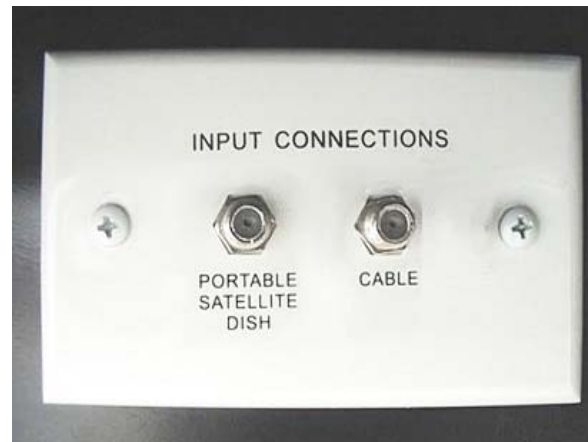
Exterior Connection for Satellite Dish and Cable TV (Located in the shoreline compartment)
