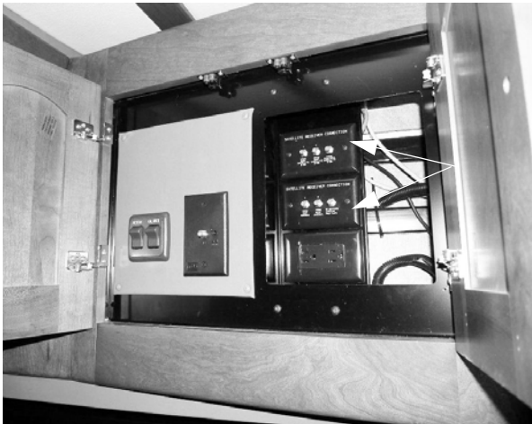
Interior Connections for Satellite Dish (Located in the overhead compartment above entrance door)
