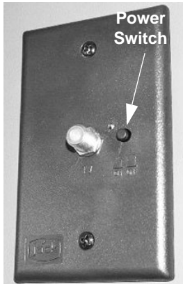
TV Signal Amplifier Power Switch (Located in overhead compartment above entrance door) -Typical View
