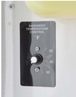
Basement Temperature Control
