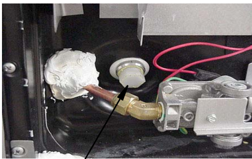
Water Heater Drain Plug (Remove with socket)
