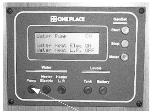
Water Pump Switch
