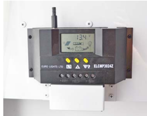
Solar Charge Controller (Located in utility compartment)
