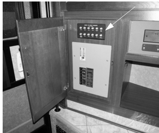
House 12-Volt Circuit Breaker Panel -Typical View
