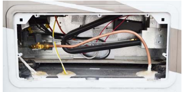
Refrigerator Access Compartment -Typical View
