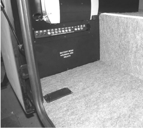
Automotive Chassis and House 12-Volt Circuit Breaker Panel (Located inside passenger compartment) -Typical View
