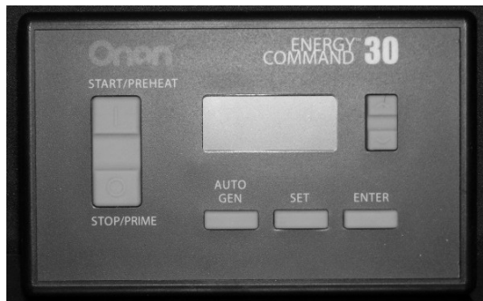
AGS Control Pad (Located near monitor panel)
