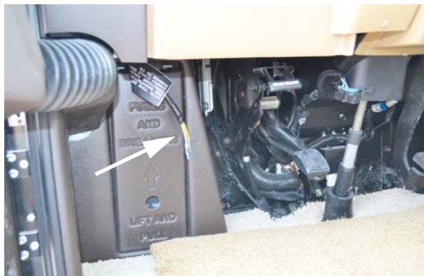
CB Power Wires (Located behind fuse and breaker panel) -Typical View
