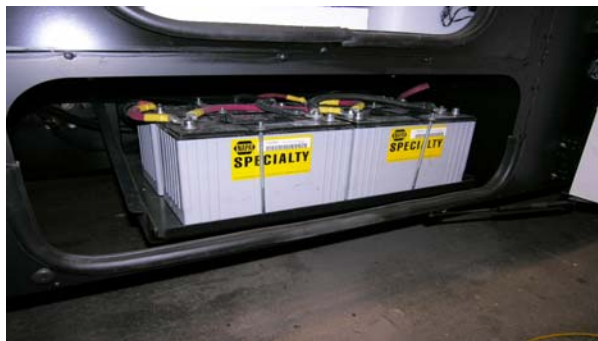
House Batteries (located in a passenger side exterior compartment) -Models 38Q and 37F
