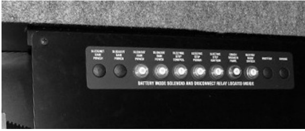
Automotive Chassis and House 12-Volt Circuit Breakers (Located inside passenger compartment) -Typical View
