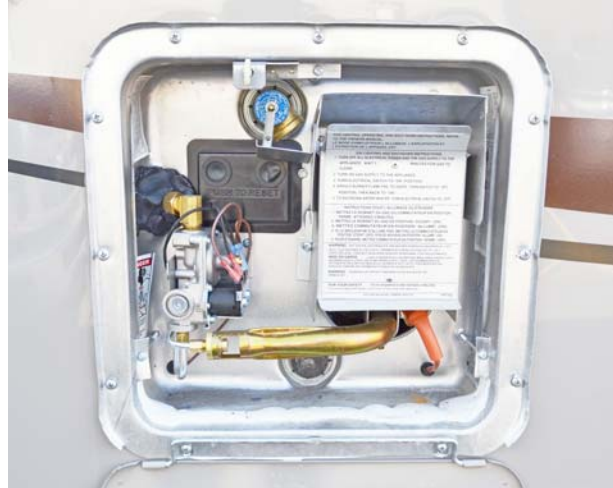
Water Heater Exterior Service Access
