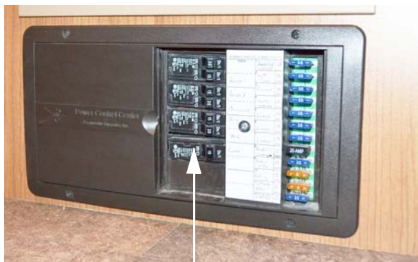
120-Volt Circuit Breakers -Typical View
