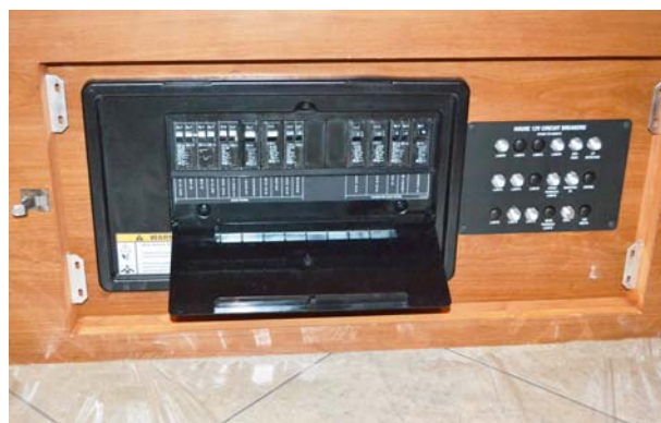
House Circuit Breakers -Typical Installation
