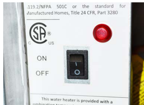
Water Heater (Tankless) Power Switch
