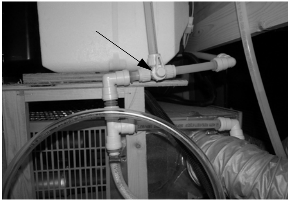
Water Heater Bypass Valve
