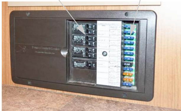
Power Center (Converter) -Typical View
