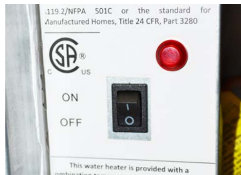
Water Heater (Tankless) Power Switch
