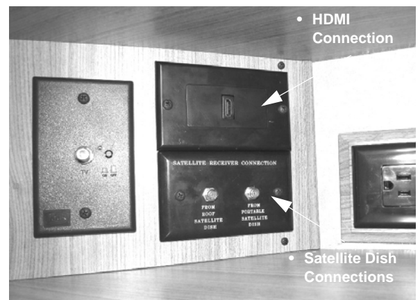
Interior Satellite Dish and HDMI Connections (Located near entertainment center cabinet) -Typical installation shown
