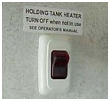
Holding Tank Heater Switch -Typical installation shown
