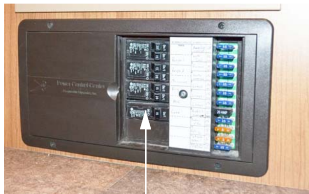
120-Volt Circuit Breakers -Typical View
