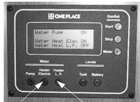
Electric LP Gas Water Heater Water Heater Switch Switch
