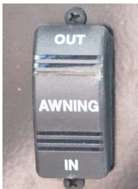
Power Awning Switch (Located near entrance door) -Typical View
