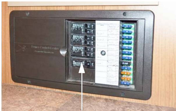
120-Volt Circuit Breakers -Typical View
