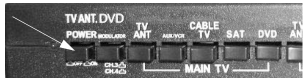
Video Selection Box (Located near entertainment center cabinet)
