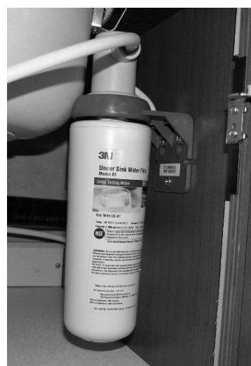
Cold Water Filter Assembly (Located below galley sink)
