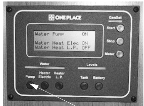
Water Pump Switch
