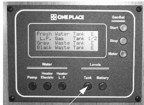
Tank Levels Switch
