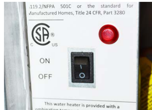
Water Heater (Tankless) Power Switch
