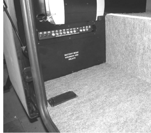
Automotive Chassis and House 12-Volt Circuit Breaker Panel (Located inside passenger compartment) -Typical View
