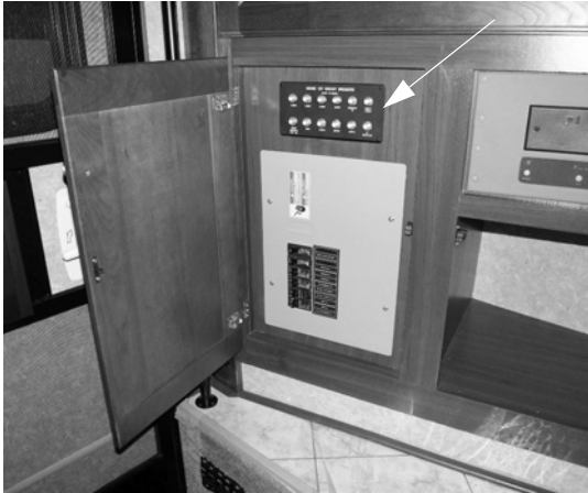
House 12-Volt Circuit Breaker Panel -Typical View
