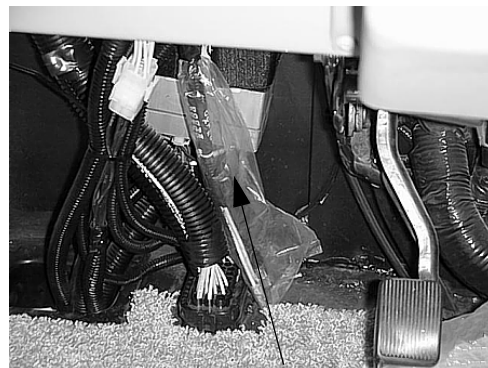
CB Power Wires (in plastic sheath) Typical View - your coach may differ
