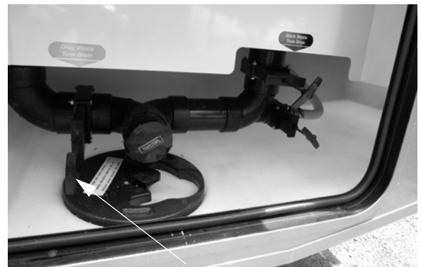
Gray Waste Tank Drain Valve (Located in water service center) -Typical View
