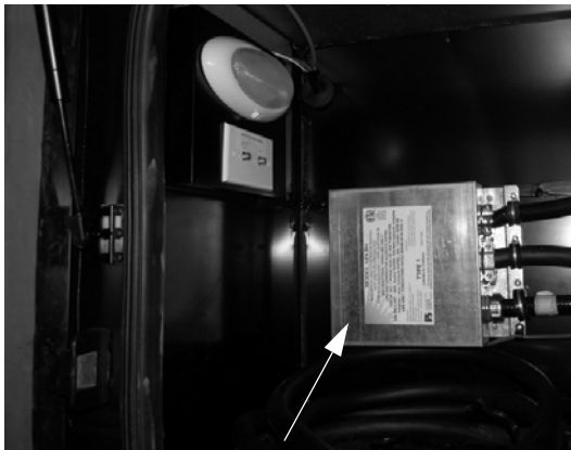
Automatic Power Transfer Box (Located inside or behind utility compartment) -Typical Installation
