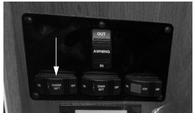
Chassis Battery Disconnect Switch (Located near entrance door) -Typical View
