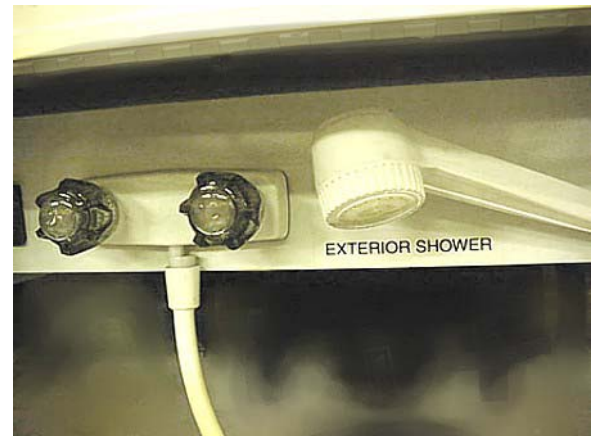
Exterior Shower/Wash Station -Typical View
