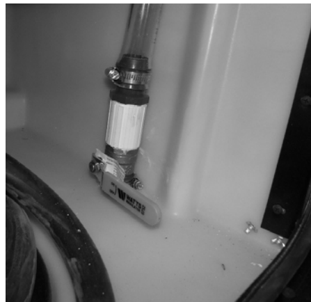
Water Tank Drain Valve (Typical)
