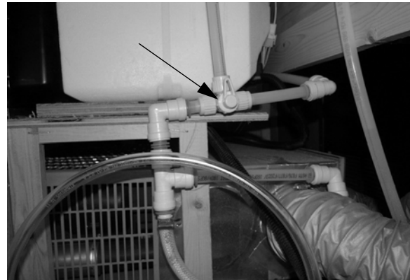
Water Heater Bypass Valve
