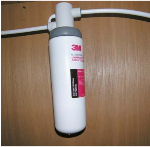
Cold Water Filter Assembly (Located below galley sink)
