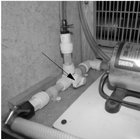
Winterization Valve -Typical View
