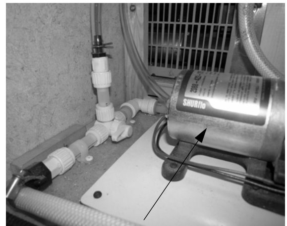
Water Pump (Located behind removable access panel in driver side rear compartment) -Typical View
