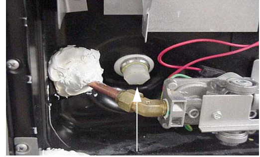
Water Heater Drain Plug (Remove with socket)
