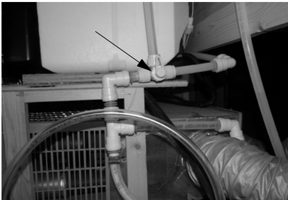
Water Heater Bypass Valve
