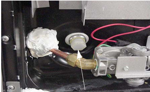
Water Heater Drain Plug (Remove with socket)
