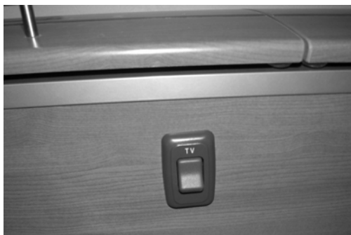
TV 12-Volt Master Power Switch (Located on underside of bedroom overhead cabinet) -Typical View
