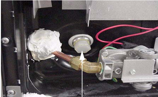
Water Heater Drain Plug (Remove with socket)
