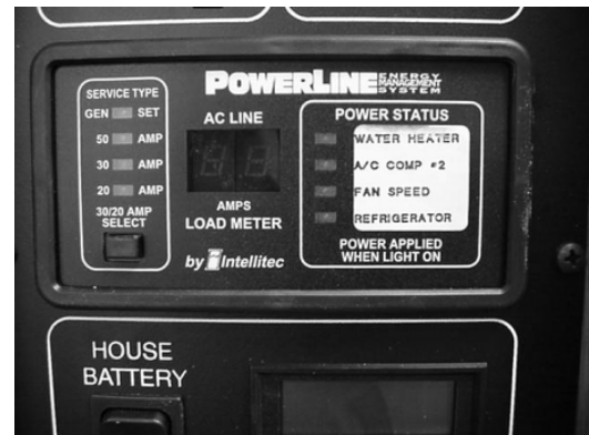
EMS Display Panel (Located on Monitor Panel) -Typical View
