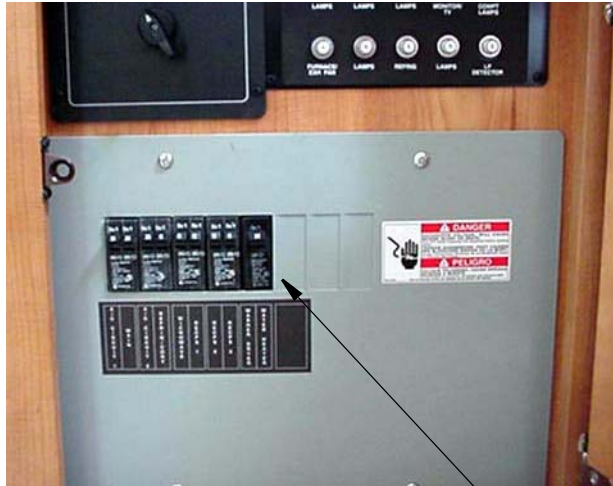
120-Volt House Circuit Breakers
