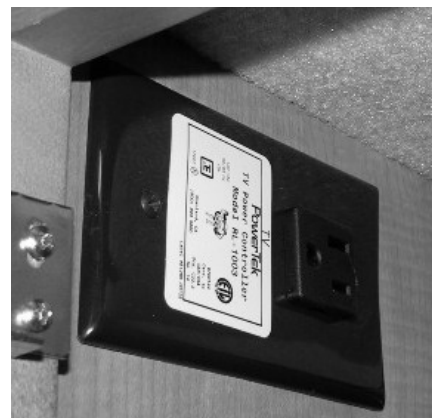
Front TV Ignition Switch Interlock -Typical View
