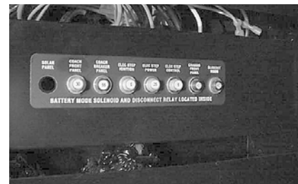
Chassis and House 12V Breakers (cover off)
