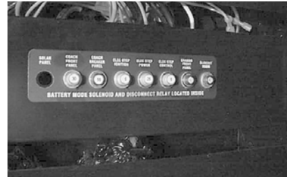
Chassis and House 12V Breakers (cover off)
