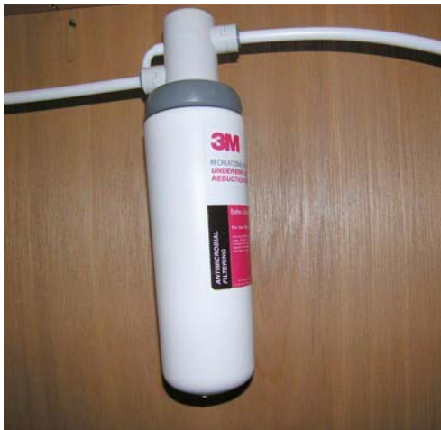
Water Filter Assembly (below Galley Sink)
