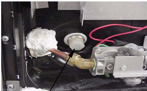
Water Heater Drain Plug (Remove with socket)
