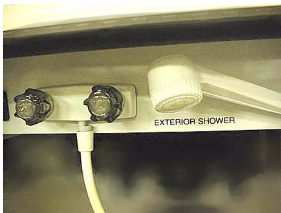
Exterior Shower/Wash Station -Typical View
