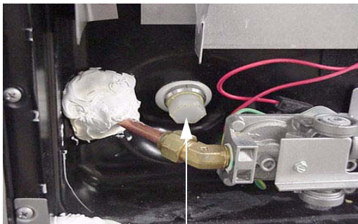
Water Heater Drain Plug (Remove with socket)
