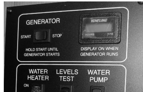
Generator Switch and Hourmeter on monitor panel
