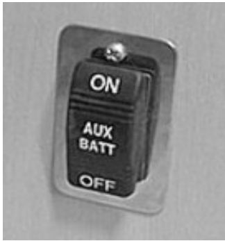
Aux. Batt. Switch - Typical (Near Systems Monitor Panel)
