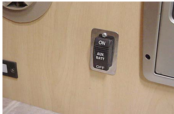
Aux. Batt. Switch - typical (Near entrance door)
