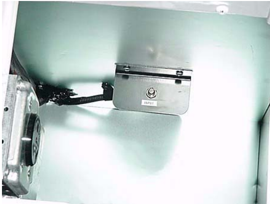
Cable TV Hook-Up in Utility Compartment
