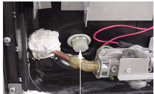
Water Heater Drain Plug (Remove with socket)
