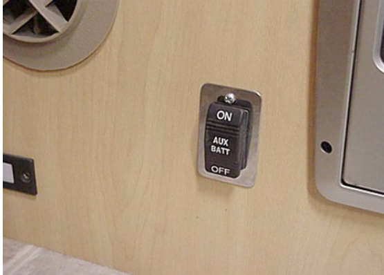
Aux. Batt. Switch (Near entrance door)
