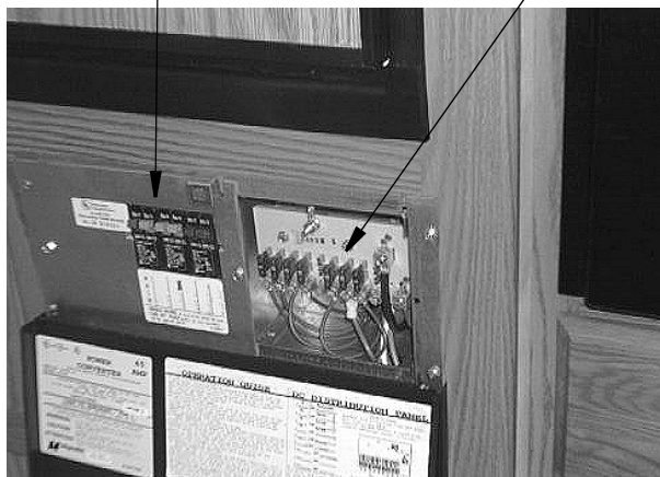
Power Center (Converter)
