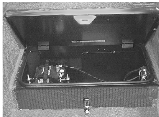
House Battery Storage in Entrance Step All Models except 322E & 322R
