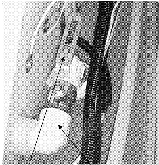
Water Tank Drain Valve Winterization Valve
